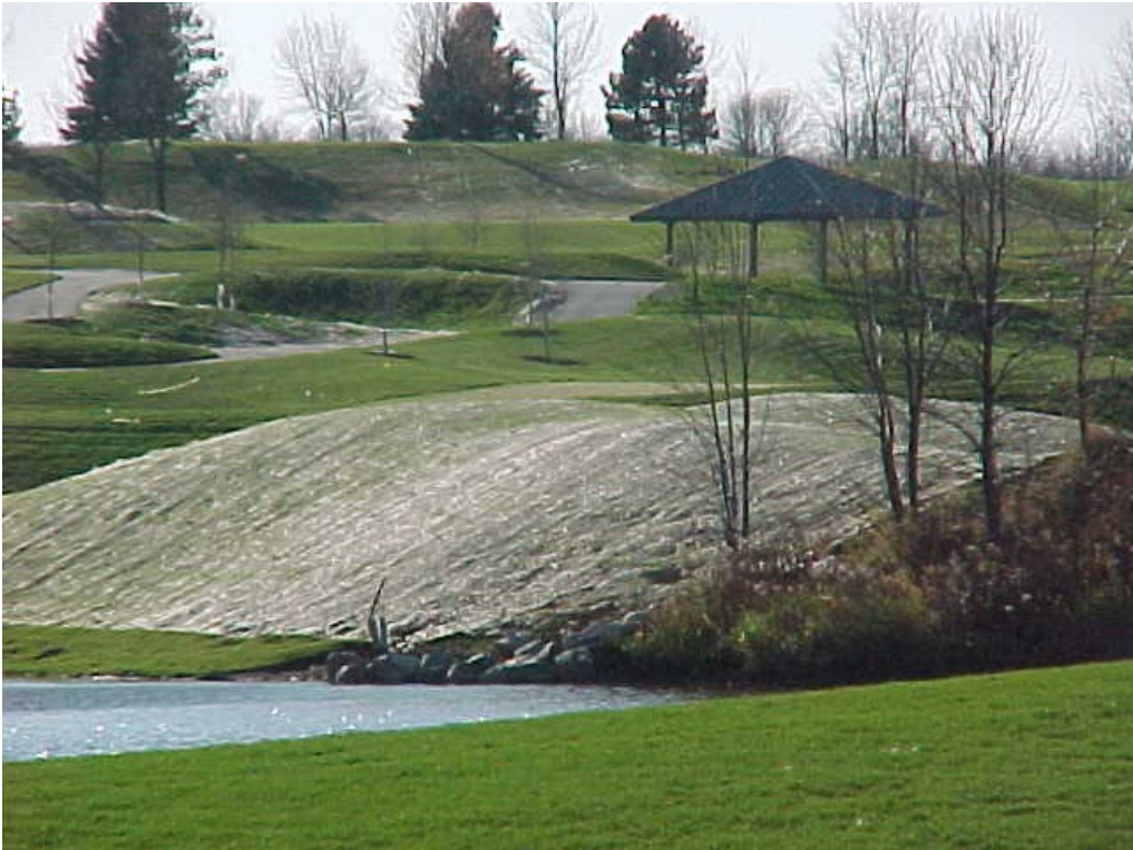
While the surrounding areas have plenty of vegetative cover, the area with erosion control blankets has around 10% vegetative cover and would not be acceptable.
