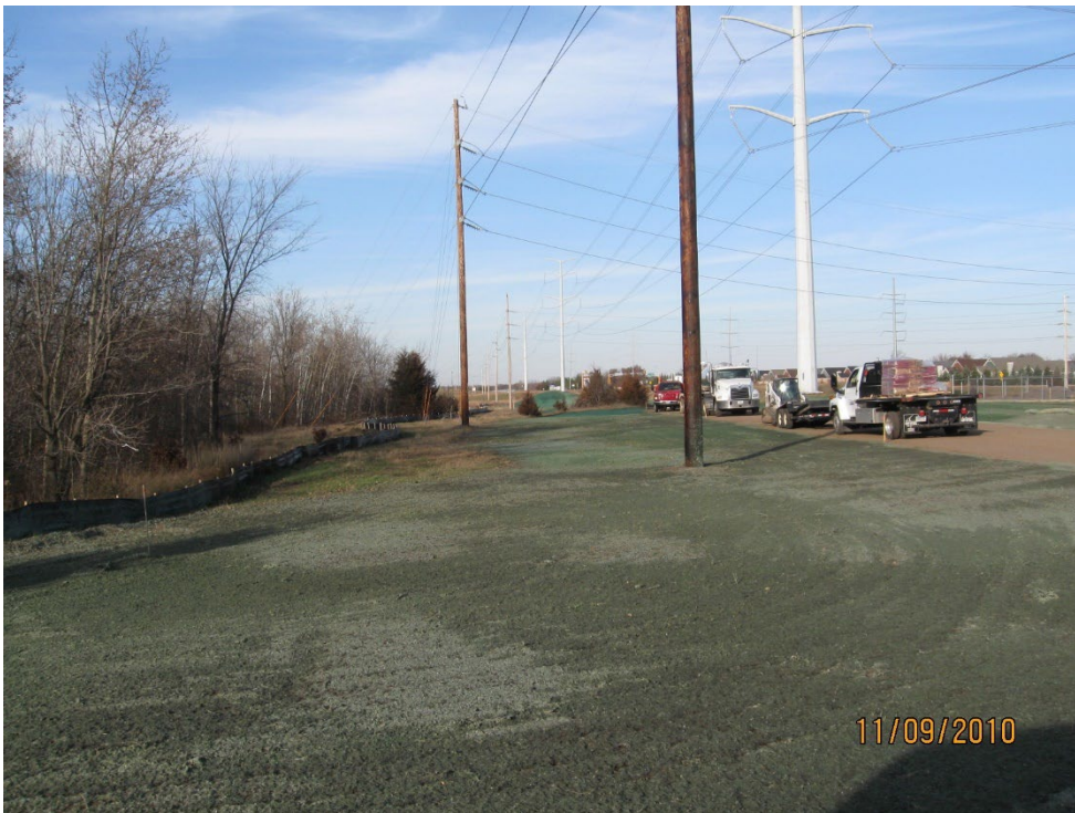
This image shows ground that has been disturbed and then stabilized with temporary hydraulically applied erosion control. This is not permanent vegetative cover and would not be acceptable.
