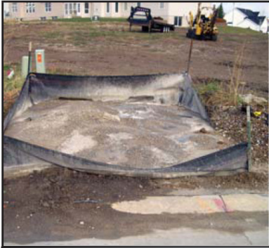
This washout needs to be maintained and is too close to the street.
